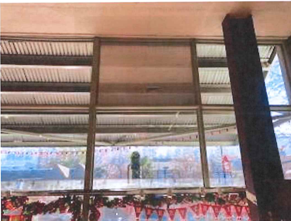
Photo D- Interior Window Panel- Inconsistent aesthetics
