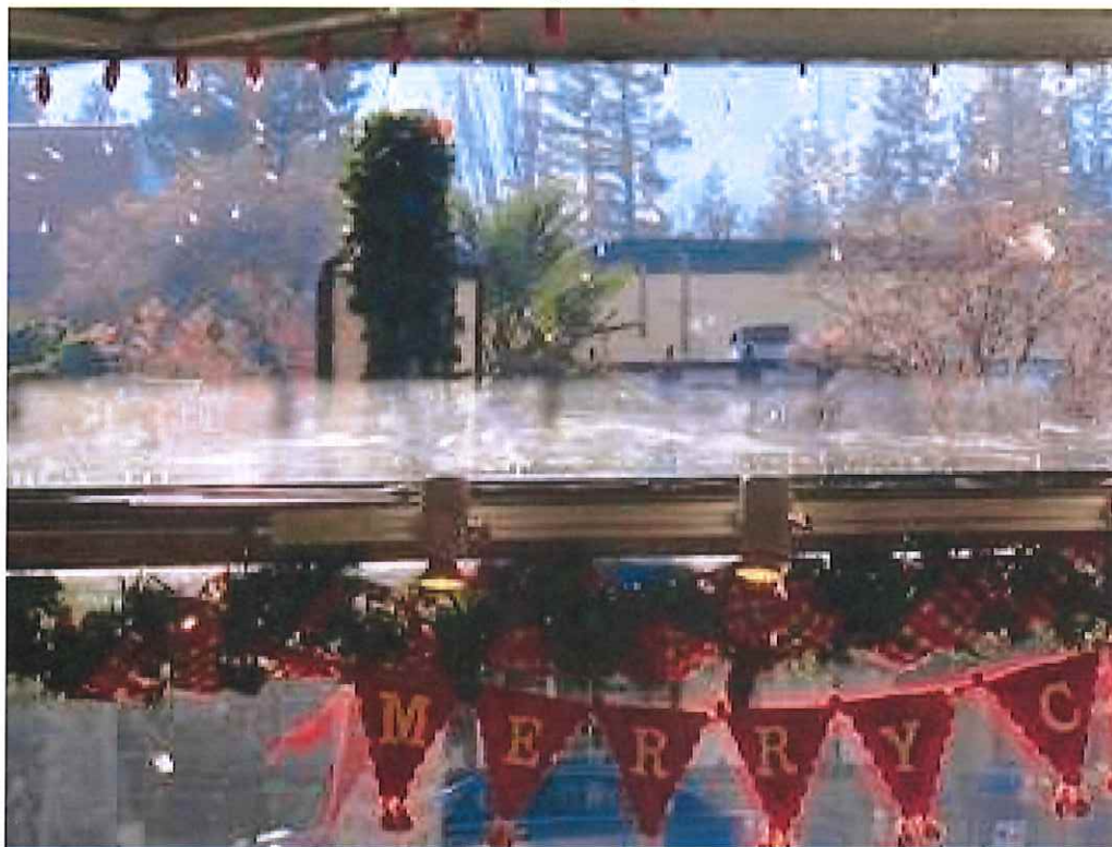
Photo F: Scratches/Wear and Tear on glass panels
