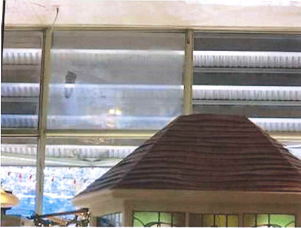
Photo A- Interior Window- Permanent Distortion
