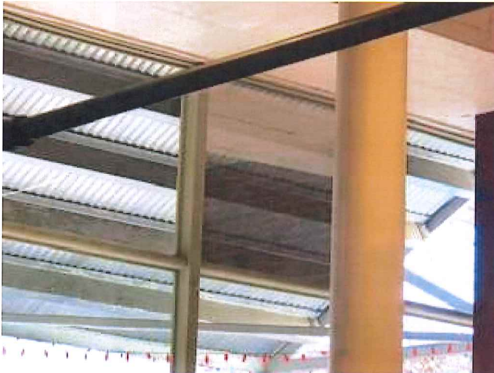
Photo B- Interior Window- Compromised window tinting, cannot be removed
