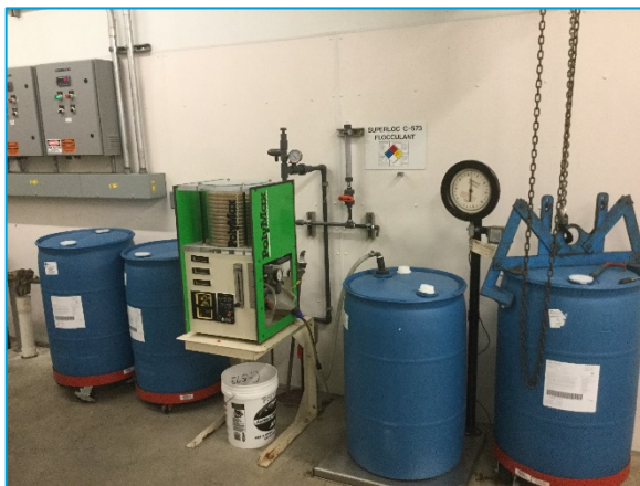
Photo 3-13 – Cationic Polymer Feeder
