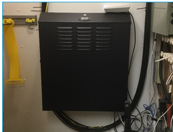
Photo 3-25 – PLC Telemetry Unit
