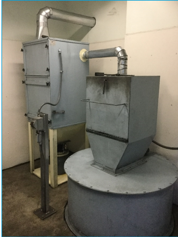
Photo 3-10 – Powdered Activated Carbon Hopper
