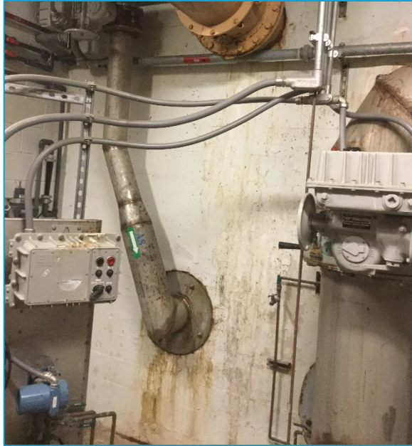
Photo 3-20 – Air Scour Air Supply (Evident Leakage)
