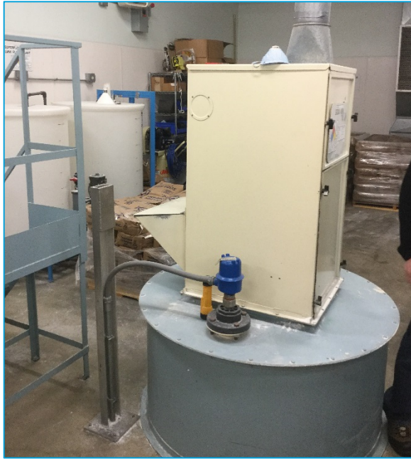
Photo 3-8 – Soda Ash Hopper
