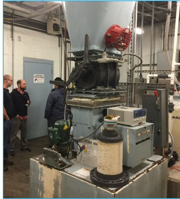
Photo 3-9 – Soda Ash Hopper, Dissolving Tank, and Metering Pumps
