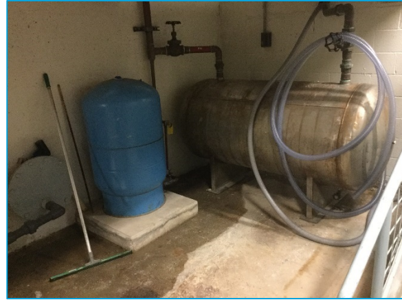
Photo 3-2 – Potable Water Storage Tank and Hydro-Pneumatic Tank
