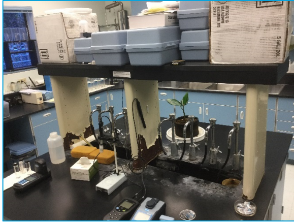
Photo 3-1 – Lab in Administration Building
