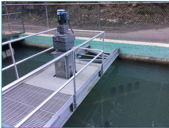
Photo 3-16 – Flocculation Basin and Paddle Mixer
