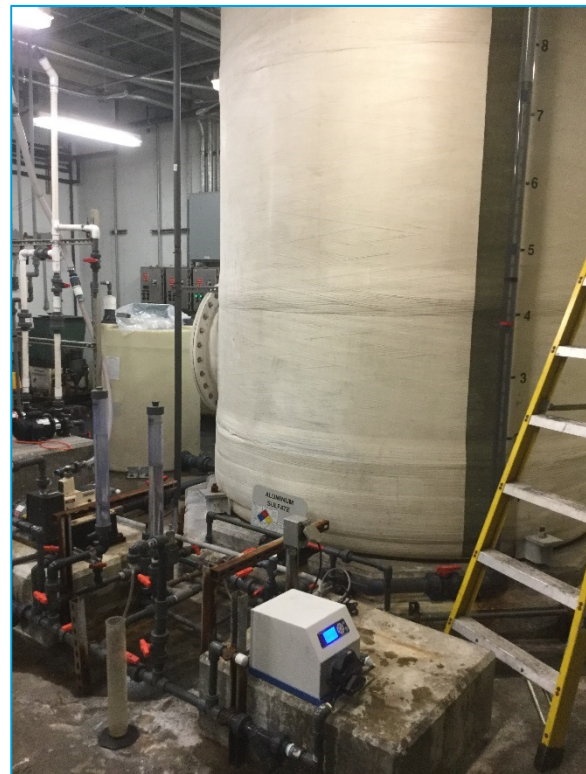
Photo 3-7 – Base and Pedestal of Alum Tank
