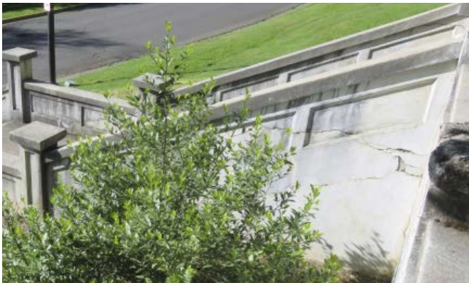
Cracks in the outer face of the staircase. This crack is also visible at the interior face.
