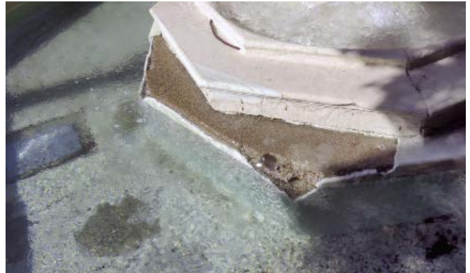
Plaster loss at concrete base. Note plaster loss below the water, on the floor of the pool.
