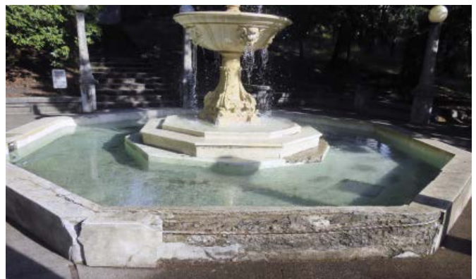
Concrete loss at outer rim of fountain pool.
