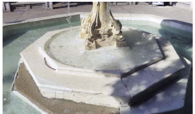
Previous repairs and open joints at lower bowl. Note the plaster failure and exposed concrete at the bottom right.
