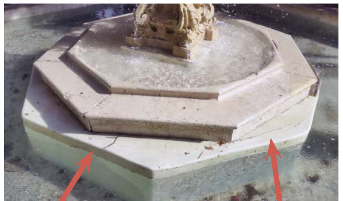
Cracks in plaster over concrete base.
