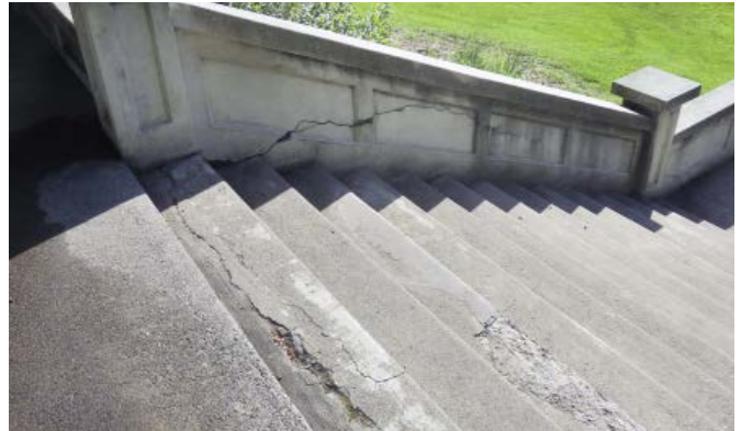
Cracks in cheek wall and failed repairs and cracks in the stairs.
