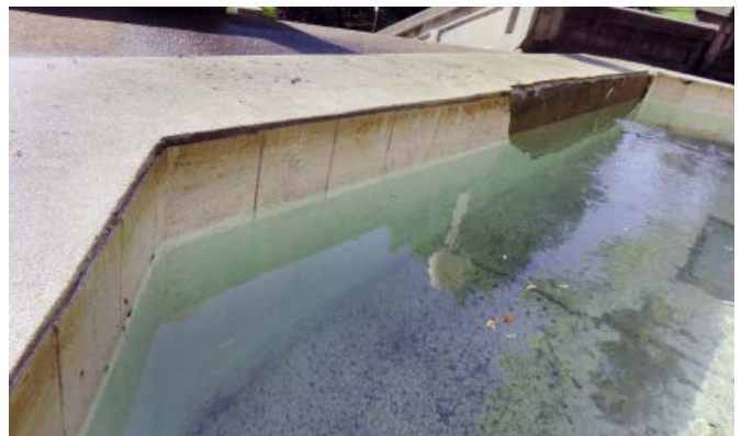
Missing and soiled perimeter tiles.
