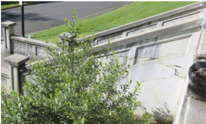
Cracks in the outer face of the staircase. This crack is also visible at the interior face.
