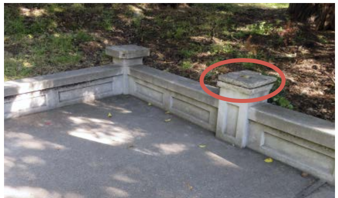
Concrete cracking, spalls, and soiling at terrace columns.
