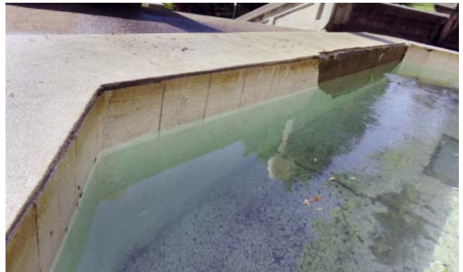
Missing and soiled perimeter tiles.
