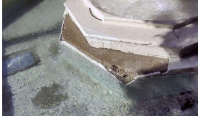
Plaster loss at concrete base. Note plaster loss below the water, on the floor of the pool.
