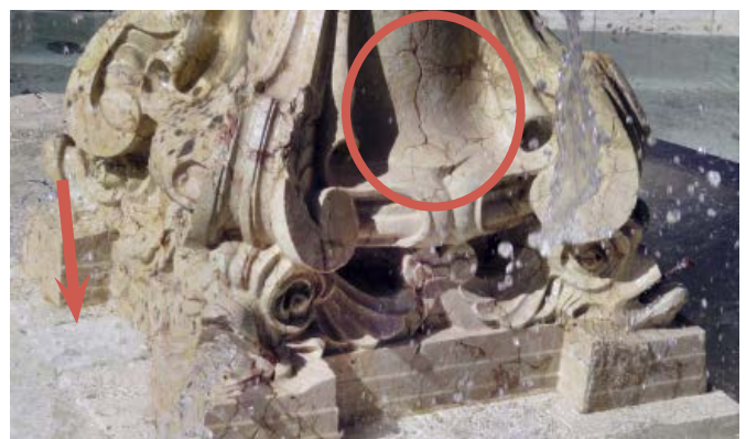
Weathered veining in lower pedestal. Note the dutchman repair indicated with an arrow.
