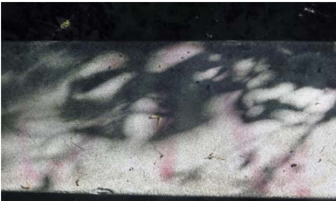
Graffiti ghosting on terrace wall.
