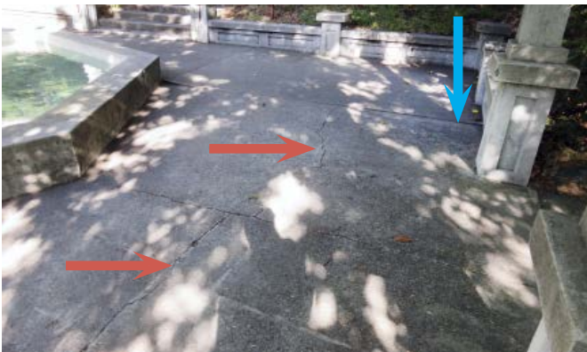
Concrete cracks (red) and warped wood strips in terrace floor (blue).
