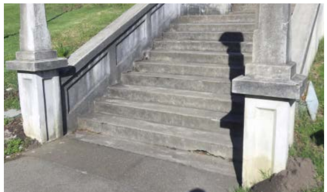
Failed repairs and small spalls at lower stairs.
