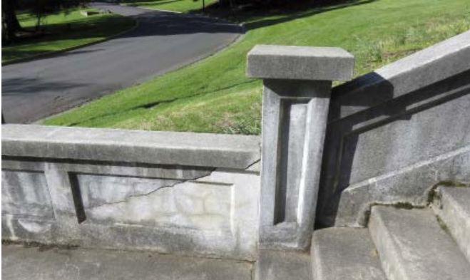
Cracks in the cheek wall. This crack is also visible at the exterior face.
