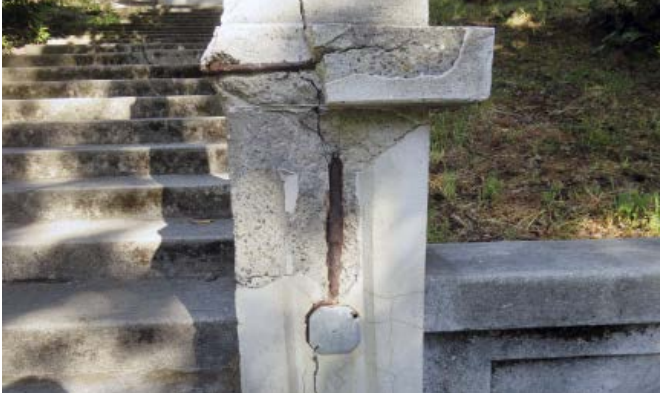
Concrete cracking and spalls at light post.
