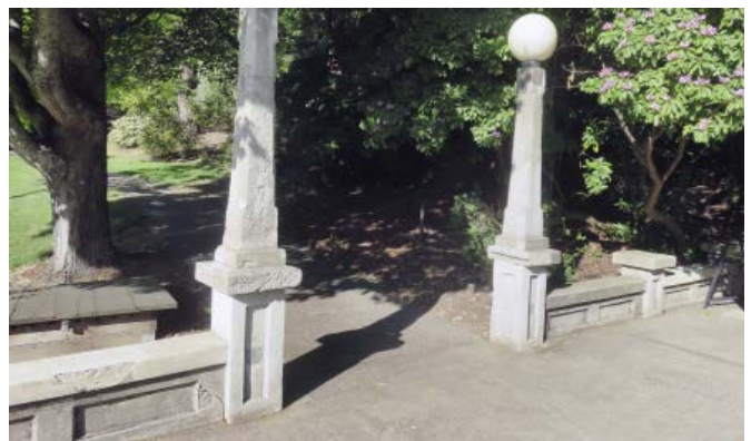
Concrete cracking, spalls, and soiling at light posts.
