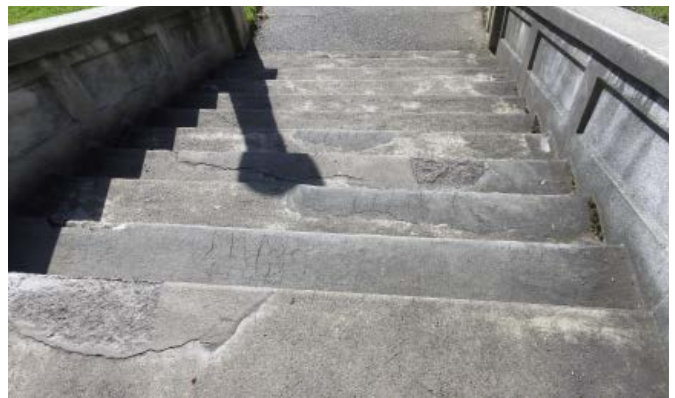
Uneven and failed repairs at the lower stairs.
