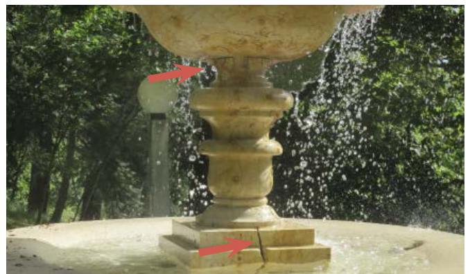
Cracks and spalls at the upper pedestal.
