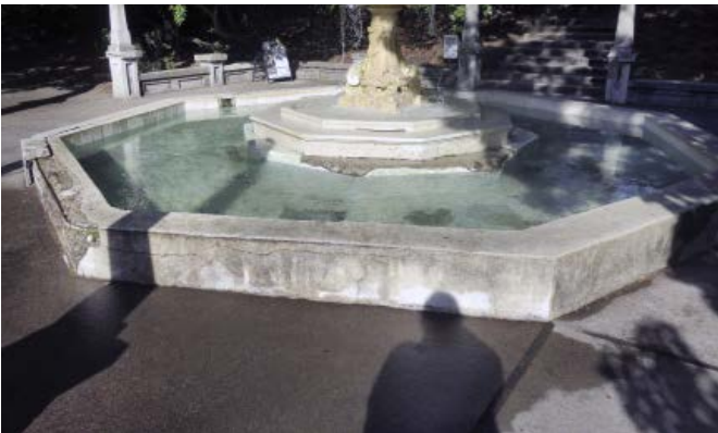
Concrete cracking, spalls, and soiling at outer rim of fountain pool.
