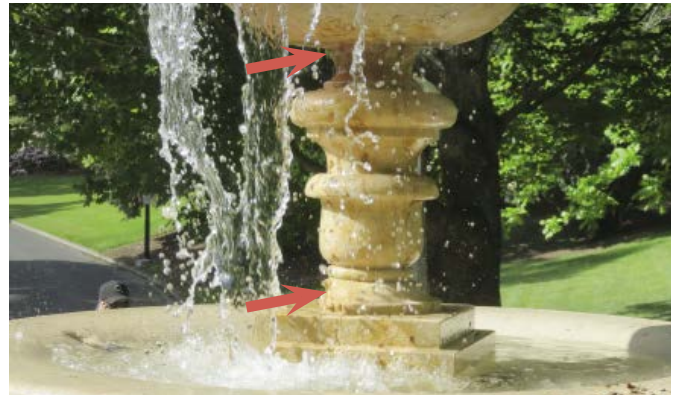
Spalls at the upper pedestal.
