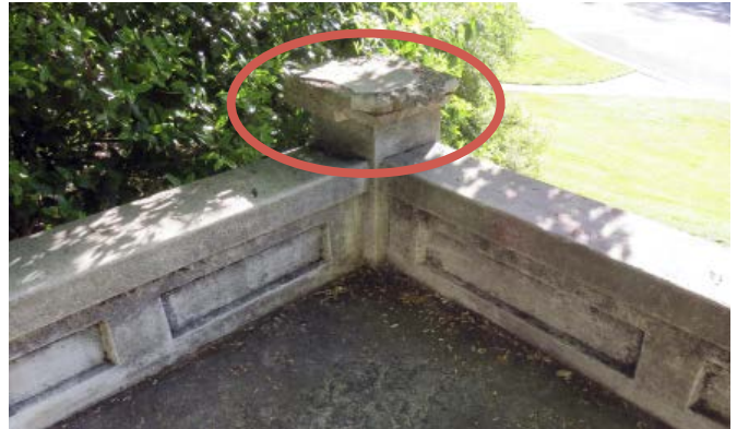
Concrete cracking, spalls, and soiling at terrace column.
