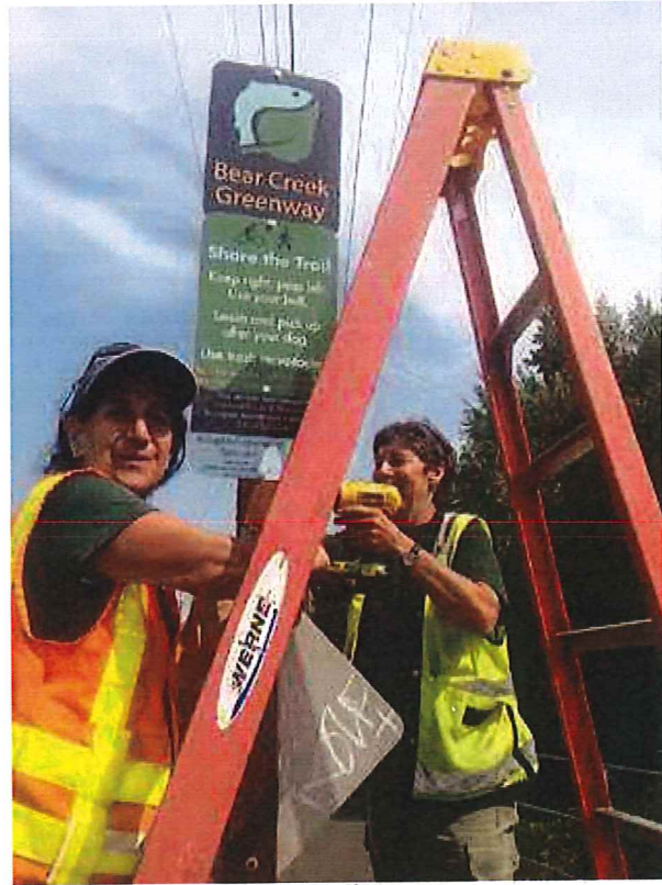
ASHLAND PARKS AND RECREATION COMMISSION SEASONAL PARK-WORKER MARIAN TELERSKI AND PARK TECH-1 TRAILS MAINTENANCE WORKER JILL MULLEN-FEELEY INSTALL NEW SIGNAGE ALONG THE ASHLAND SECTION OF THE BEAR CREEK GREENWAY TRAIL.
