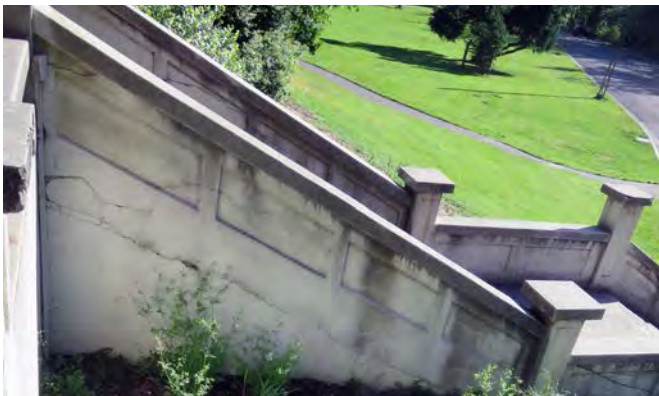
Cracks in the outer face of the staircase.
