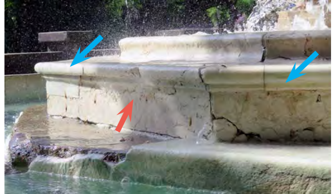
Crack (red) and dutchman repairs (blue) in lower bowl. Note the open joint between the plaster and the marble.
