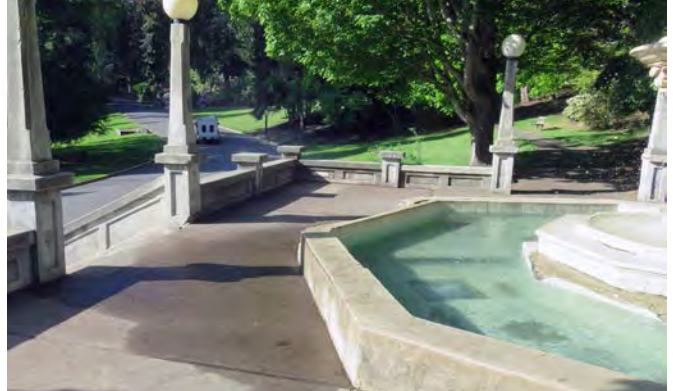
Water splashes out of the east end of the fountain, at the top of the stairs.
