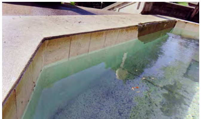
Missing and soiled perimeter tiles.
