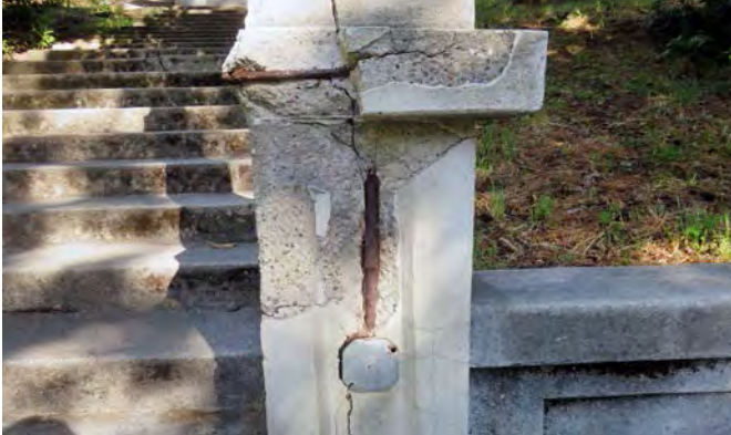
Concrete cracking and spalls at light post.
