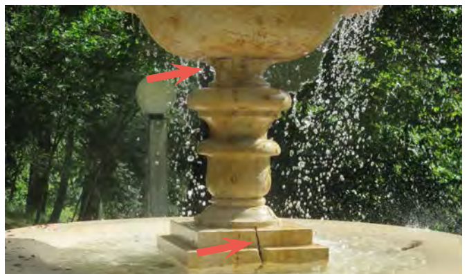
Cracks and spalls at the upper pedestal.
