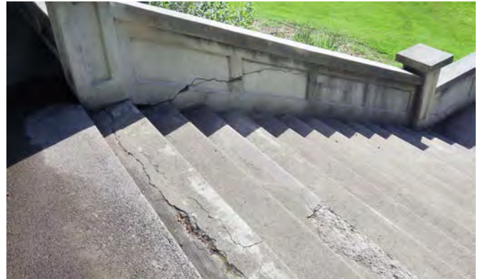
Cracks in cheek wall and failed repairs and cracks in the stairs.
