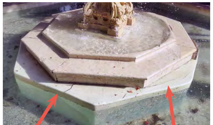
Cracks in plaster over concrete base.
