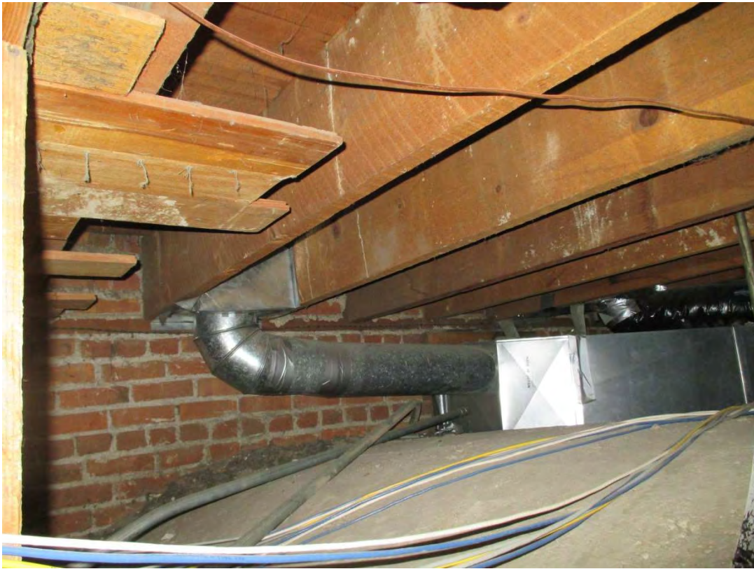
PHOTO 0236 – Upper floor framing visible in the main floor ceiling cavity adjacent to a vault
