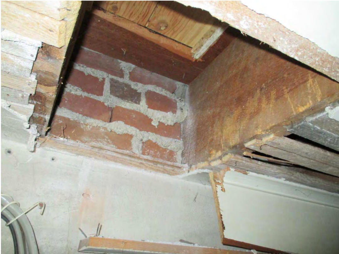
PHOTO 0242 – Upper floor connection at the east URM wall of the main building area
