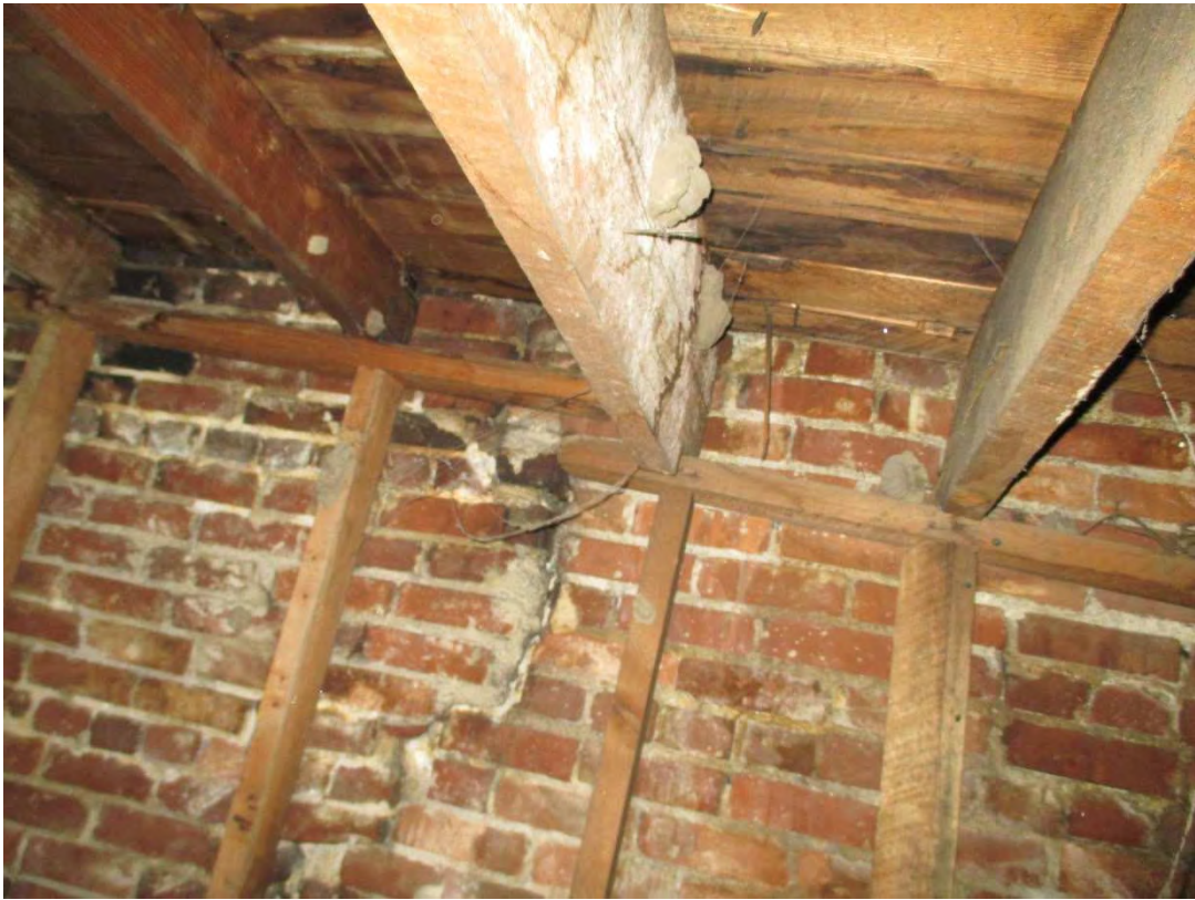
PHOTO 0254 – Joint at the east wall between the 1891 building to the south and the 1913 addition
