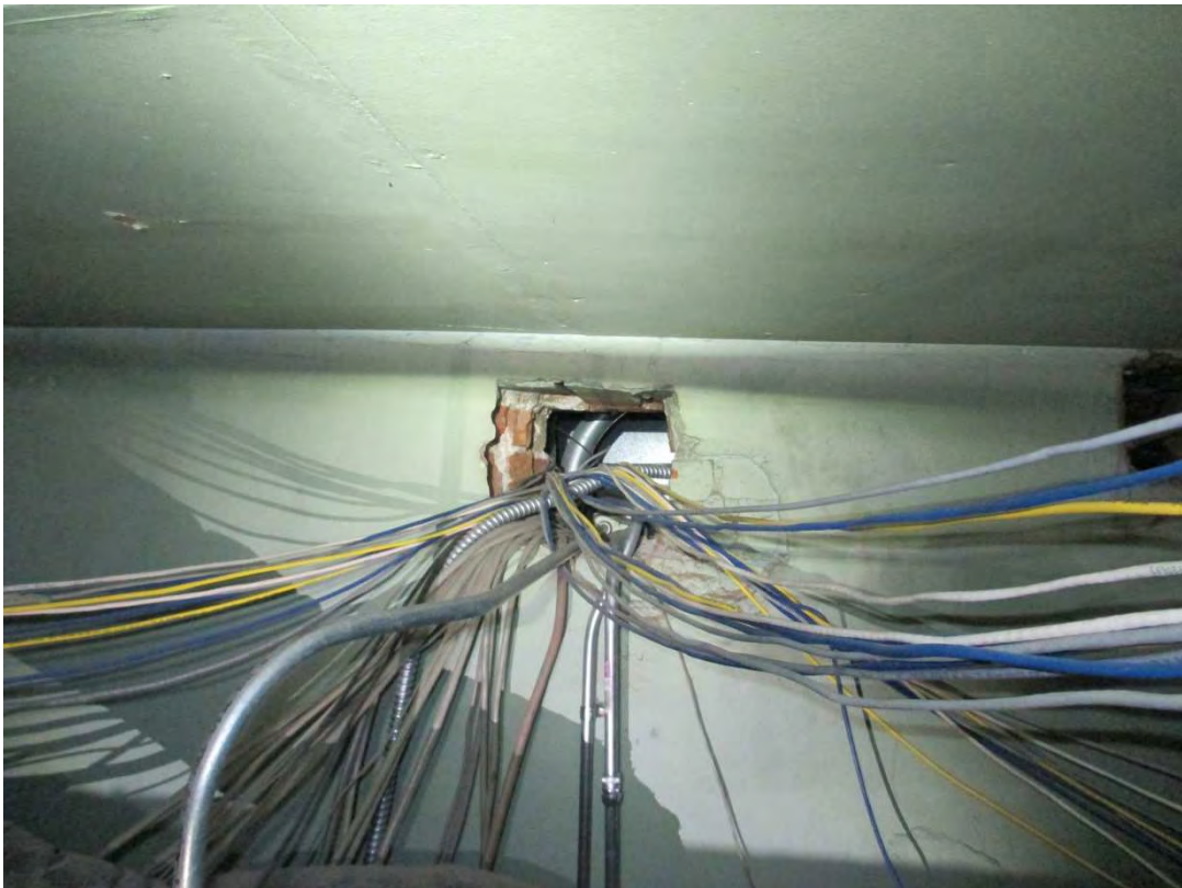
PHOTO 0235 – Access opening through the east URM wall in the main building area
