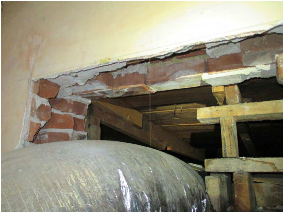
PHOTO 0261 – HVAC access in the upper floor ceiling cavity through the east wall
