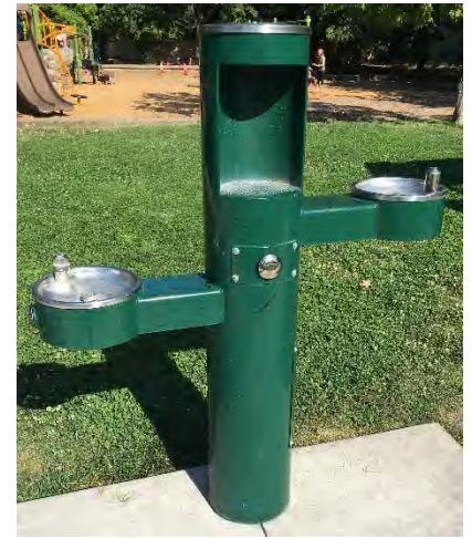
Fig. 3 - Newly installed ADA fountain with bottle filler at Garfield Park
