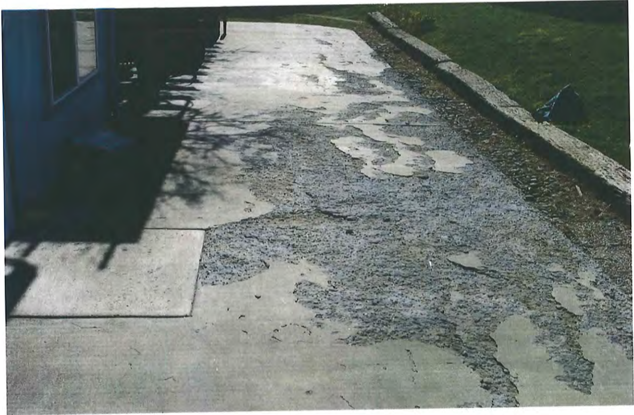
Crumbling concrete patio
