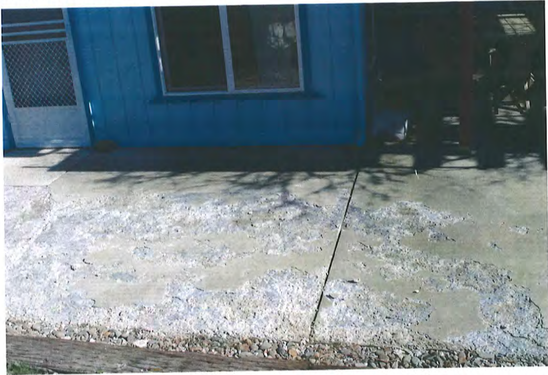
Crumbling concrete patio. Laundry room add-on to be demolished.
