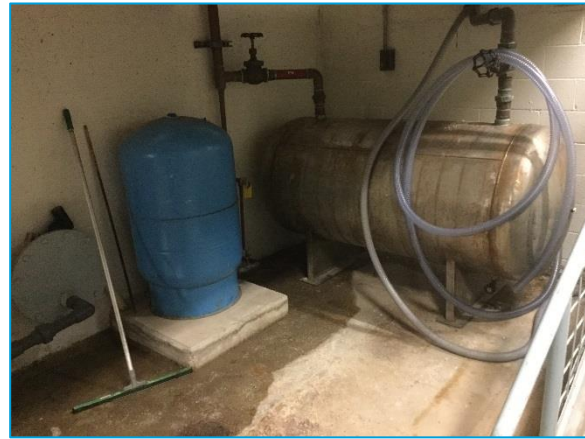
Photo 3-2 – Potable Water Storage Tank and Hydro-Pneumatic Tank
