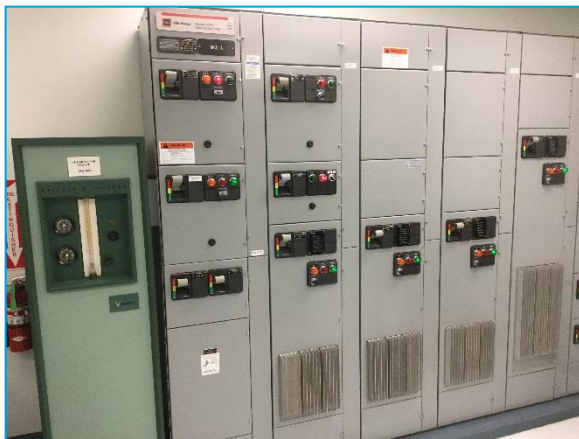
Photo 3-22 – Motor Control Center
