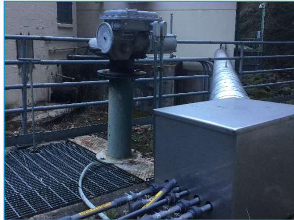
Photo 3-4 – Influent 36-inch Butterfly Valve
