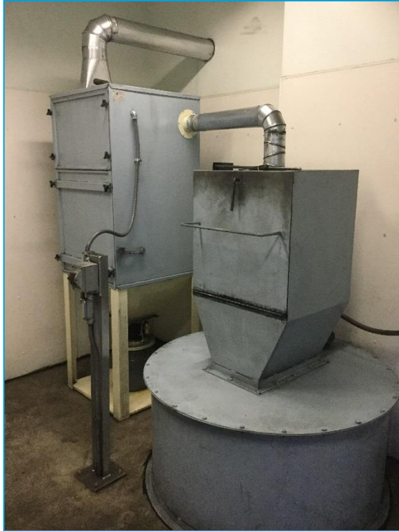
Photo 3-10 – Powdered Activated Carbon Hopper
