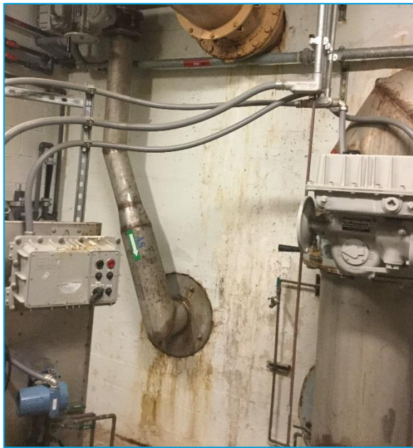
Photo 3-20 – Air Scour Air Supply (Evident Leakage)
