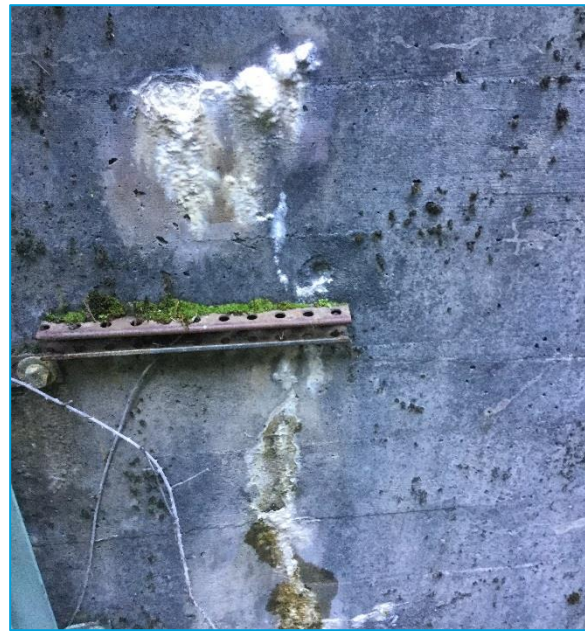
Photo 3-21 – Efflorescence on Exterior Dual Media Filter Wall
