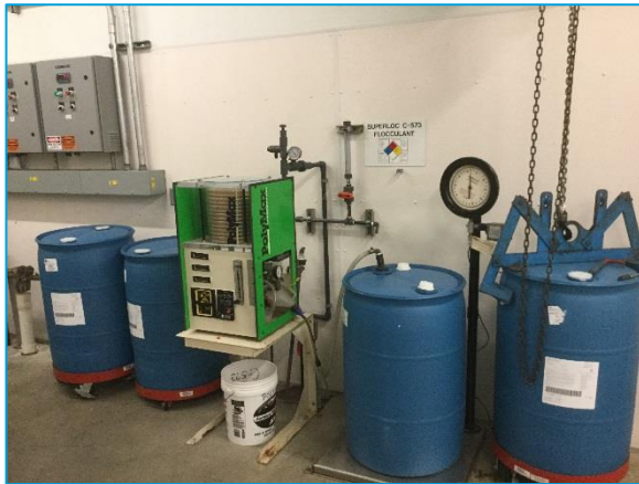
Photo 3-13 – Cationic Polymer Feeder
