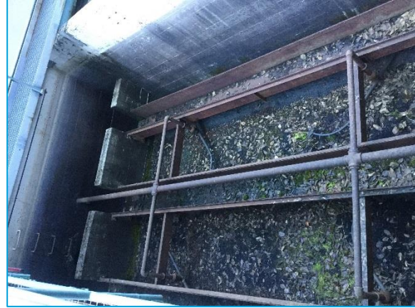
Photo 3-19 – Abandoned Dual Media Filter #7
