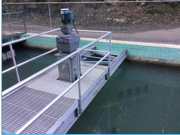
Photo 3-16 – Flocculation Basin and Paddle Mixer
