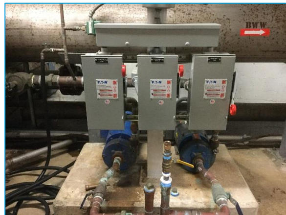
Photo 3-23 – Potable Water Pump Disconnects
