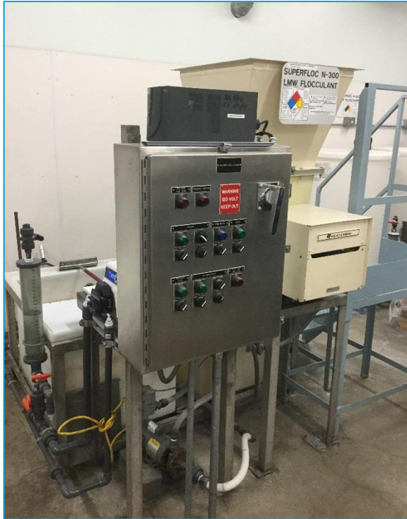
Photo 3-11 – Filter Polymer Aid Hopper and Mixing Tank
