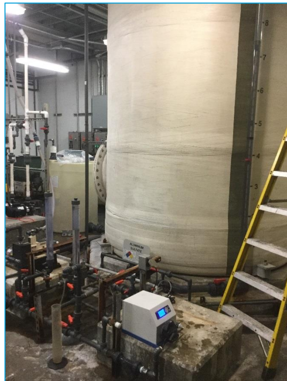
Photo 3-7 – Base and Pedestal of Alum Tank
