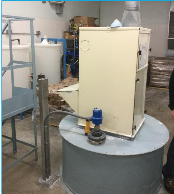
Photo 3-8 – Soda Ash Hopper
