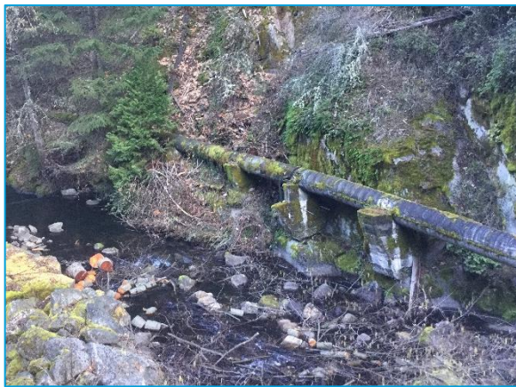
Photo 3-5 – Talent Irrigation District Influent Pipeline
