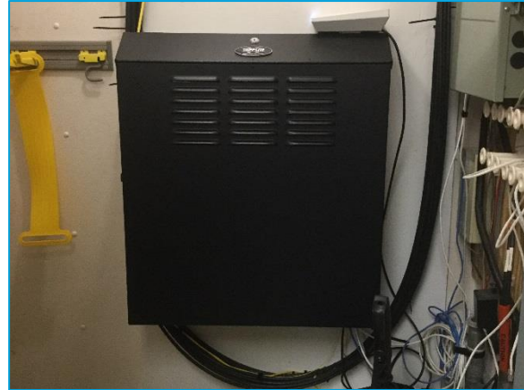
Photo 3-25 – PLC Telemetry Unit
