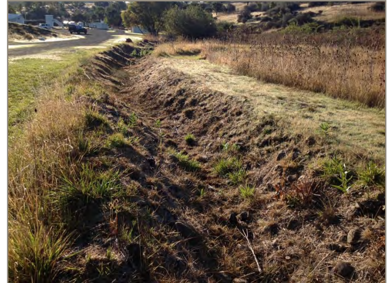
Photo 20: View of the east end of a ditch between Wetland 1 and a road, originating at the junction with the main access road.
