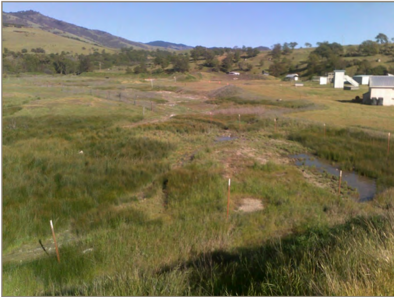
Photo 1: Filling, grading and berm construction seen for Gun Club purposes. Photo overlooking Wetland 3.
