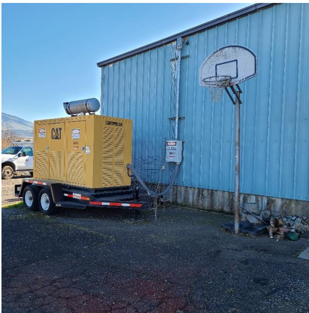
Existing generator at the Talent BPS
