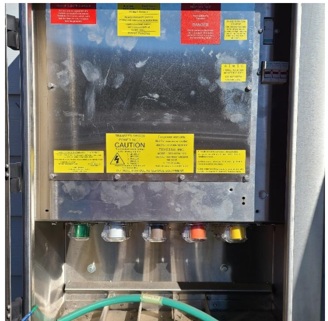
BPS generator electrical power inlet cabinet
