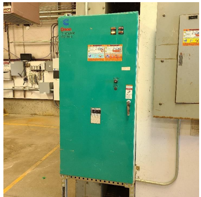
Existing automatic transfer switch in Talent BPS
