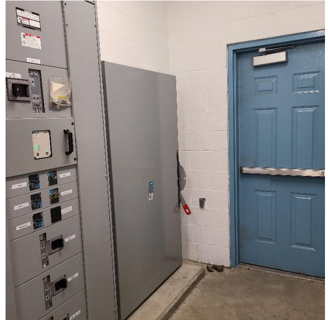
Manual transfer switch inside Ashland BPS
