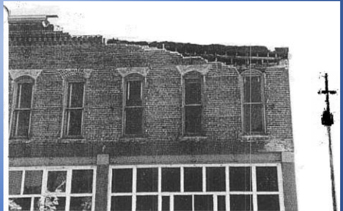
Figure 3 - The Stevens Building lost part of its parapet and wall, and suffered large shear/flexural cracks in the storefront brick piers.
