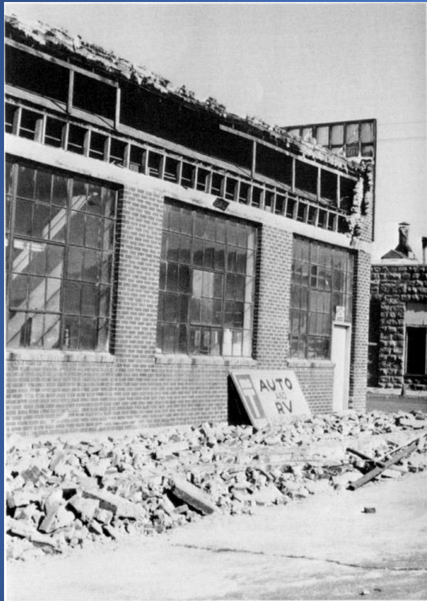
Klamath Falls, Oregon, earthquakes on September 20, 1993. Fallen debris litter the sidewalk beneath a partially collapsed, unreinforced-masonry wall and parapet in downtown Klamath Falls.
