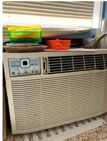
Image 2: Example of Packaged AC unit
