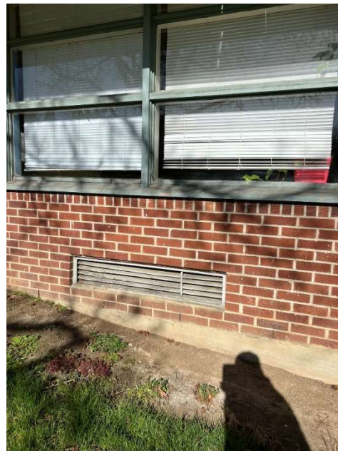
Image 10: Exterior fresh air louver
