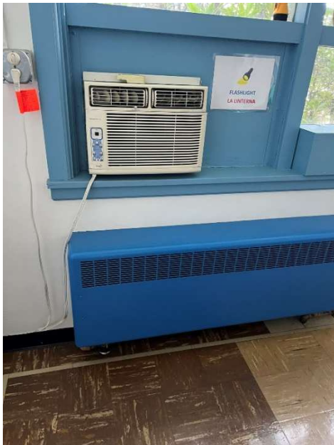
Image 9: Radiant heater and Packaged AC
