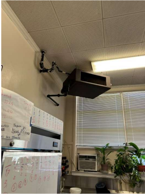
Image 7: Ceiling mounted radiant heater
