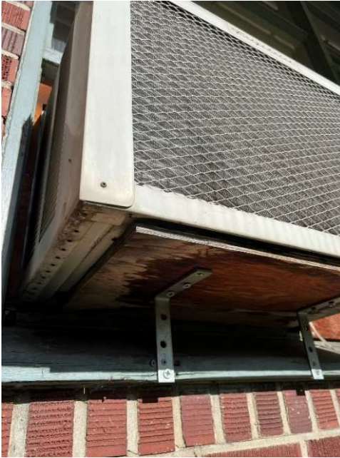
Image 3: Exterior of Packaged AC unit
