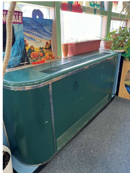
Image 6: Radiant heater in classroom
