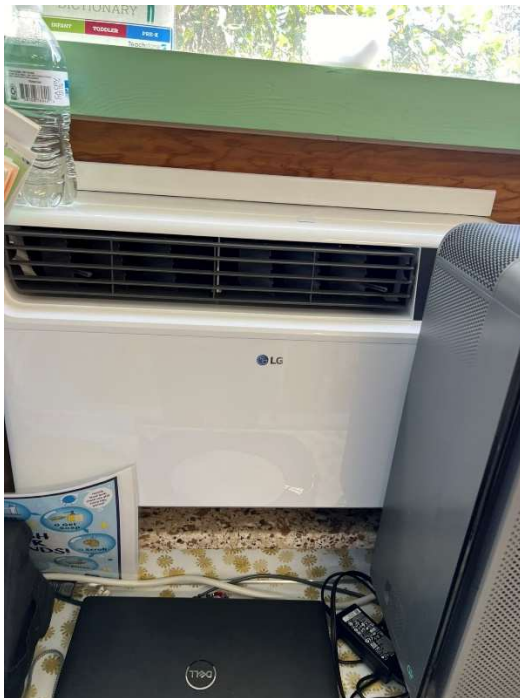
Image 5: Interior packaged AC unit
