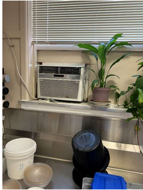
Image 4: Interior Packaged AC unit
