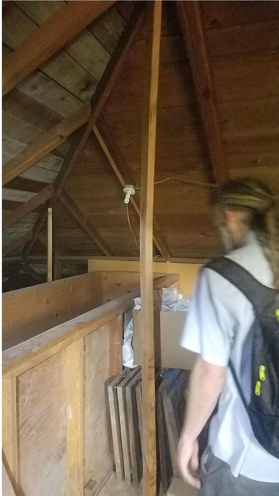
Figure 3. Winburn Way Community Center, Over-stressed hip support
