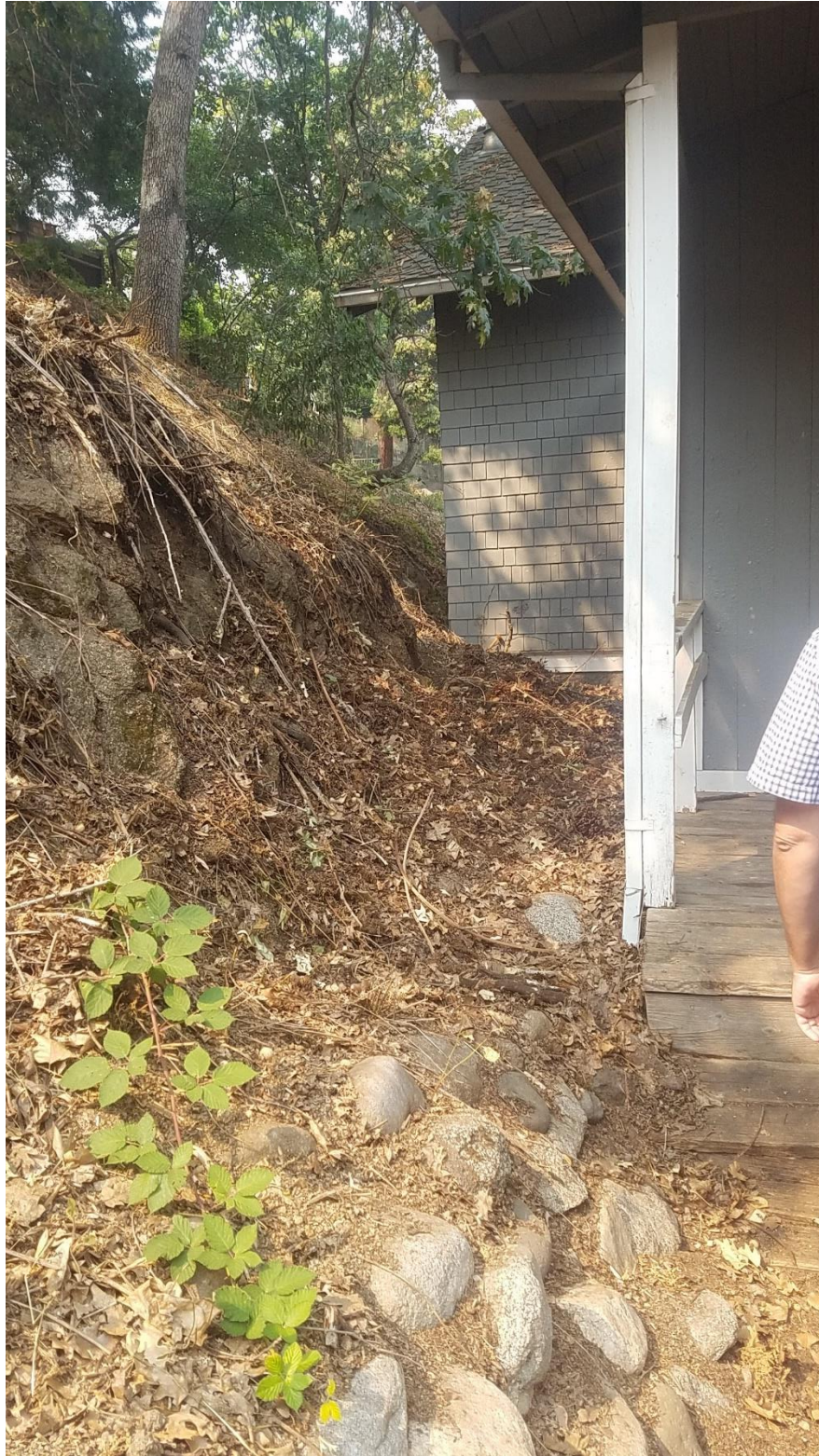
Figure 4. Winburn Way Community Center, Rear Sloughing Conditions
